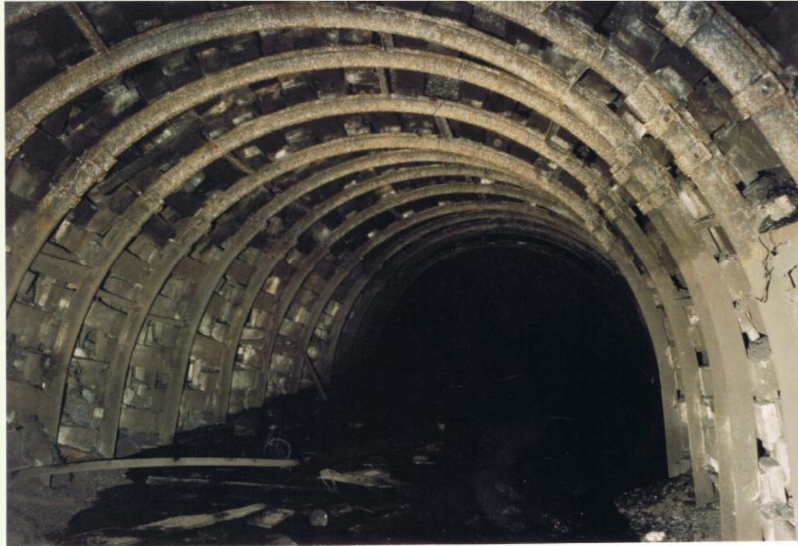
4 x-cut East Return, intersection to east of Vent Shaft (half full of water)
